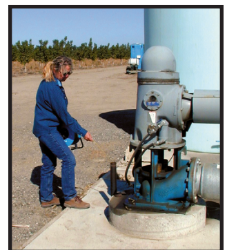
Figure 3. Measuring the depth of water table in an irrigation well with an electric well sounder. Note pipe provides entry into well casing.
