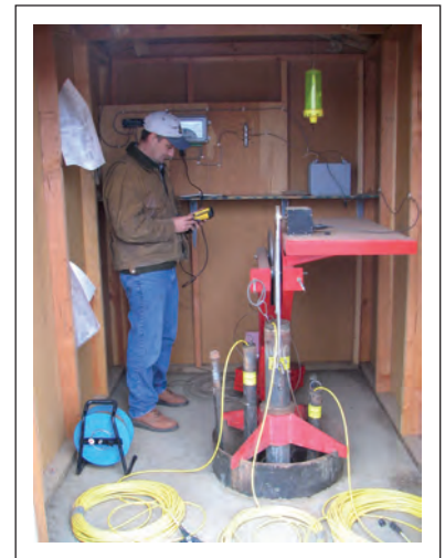
Figure 4. Above-ground portion of a cable extensometer with recording equipment.
