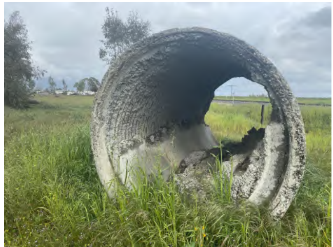
View of concrete debris.
